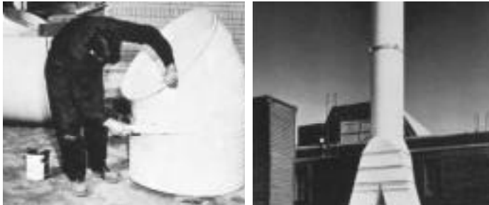
Corrosive Fumes Installation
